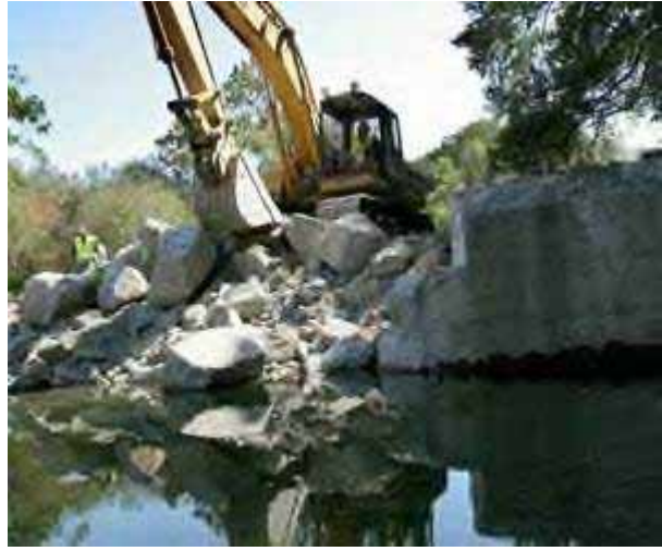
AN EXCAVATOR prepares to haul the crumbled remains of the Sunol Dam from the Alameda Creek near Sunol on Thursday. Today, the San Francisco Public Utilities Commission will remove the last of the dam, opening the creek to steelhead and salmon runs for the first time in 100 years. (Nicole Hill - Staff)
