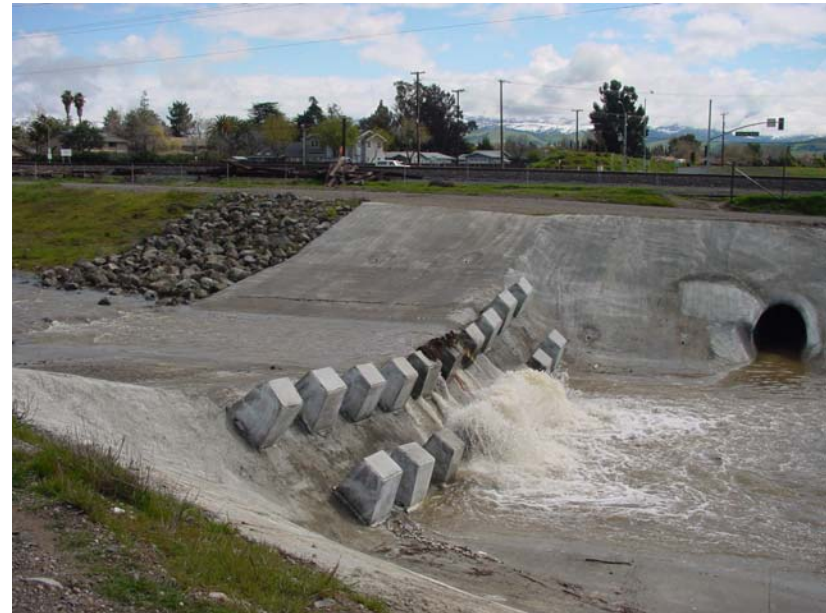
Gradient structures just before and after Isabel overcrossing
