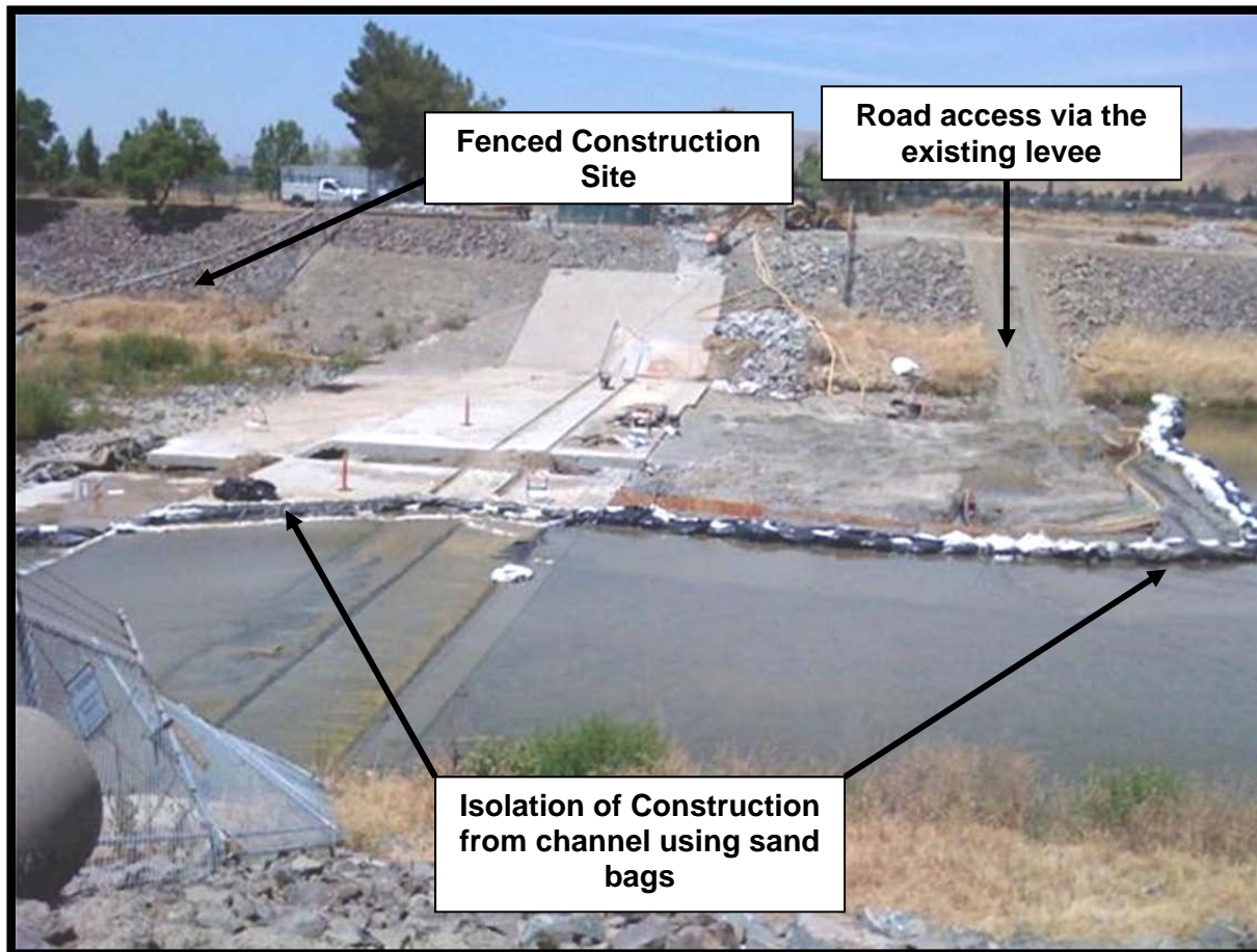
Figure 10. Typical site isolation and construction zones (per the previous ACWD removal of Rubber Dam 2).
