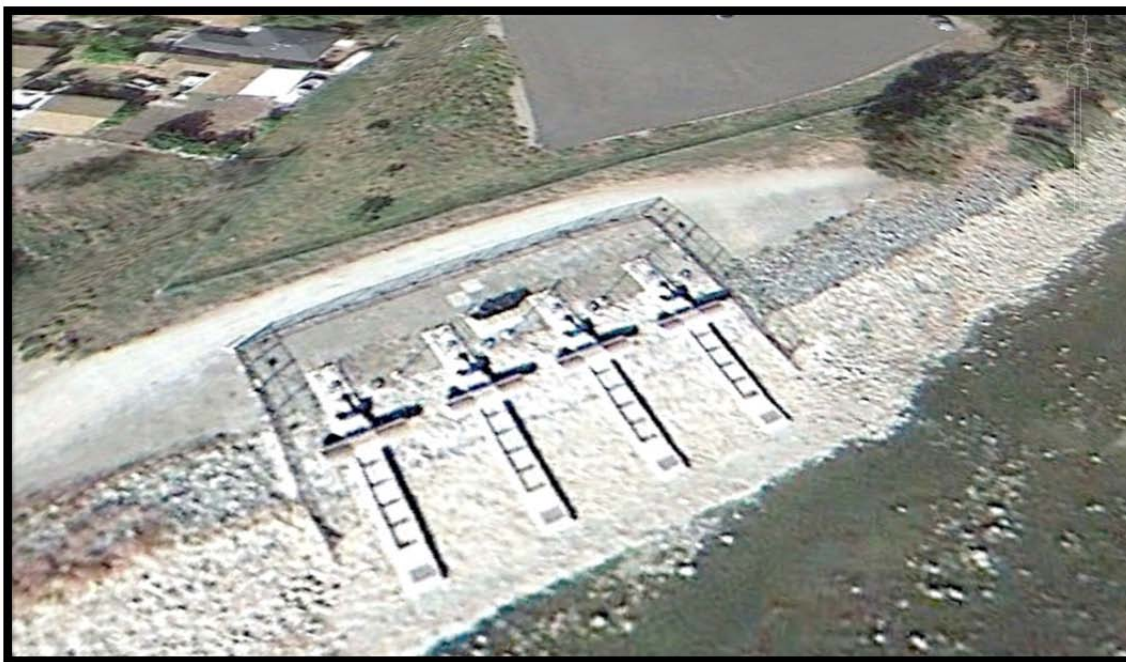
Figure 7. Existing fish screens upstream of Rubber Dam 3. The consolidated Shinn Pond Screens will be similar in configuration.
