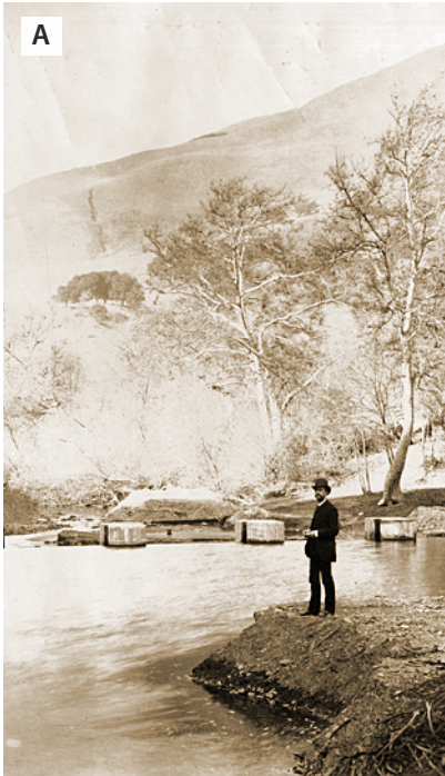
Figure 5.13. Sunol Dam. Sunol Dam was constructed in 1900 (A; shown under construction) to trap water from Alameda Creek in the Sunol filter galleries. Previously, water had been diverted further downstream at the Niles Dam. (B) Floodwaters flowing over Sunol Dam. (A: #158383, © San Francisco Public Utilities Commission; B: from SVWC ca. 1900-29, courtesy The Bancroft Library, UC Berkeley)
